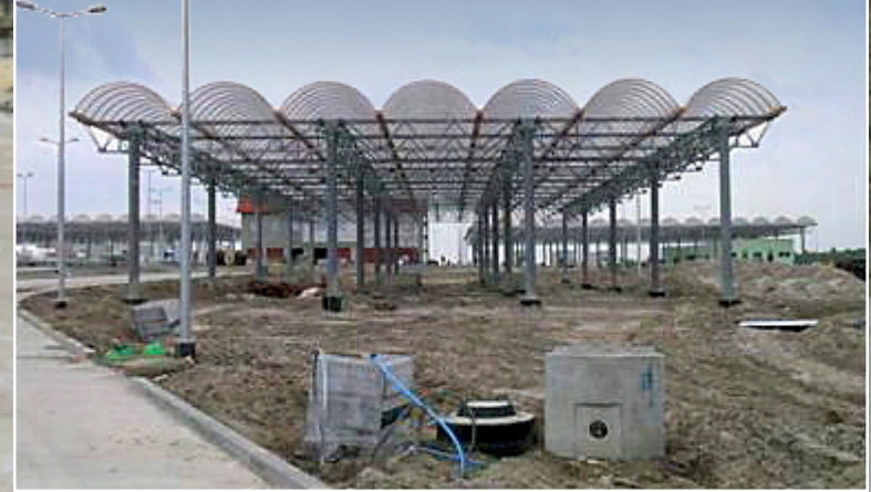
View of the clearance lines under construction at the Road Border Crossing in Hrebenne (June 2005)
