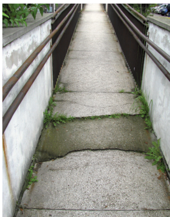
Picture 5 Poor state of slipways impeding the motion of a wheelchair
