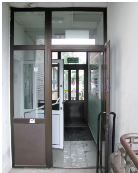
Picture 4 Entry door impeding wheelchair access
